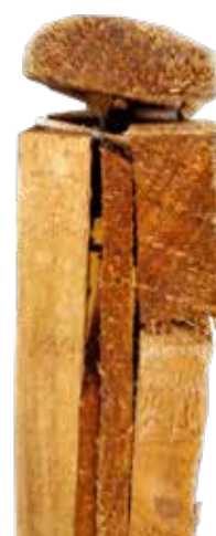
Capping rail 'popping off'
